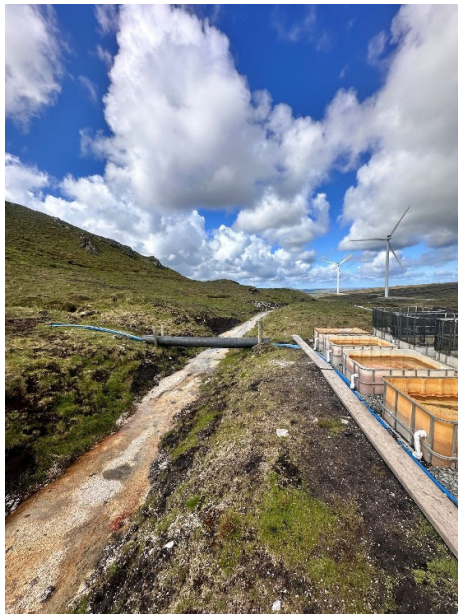
Photo 5. Existing drainage treatment system (left) and pilot trials (right) north of KBP02
