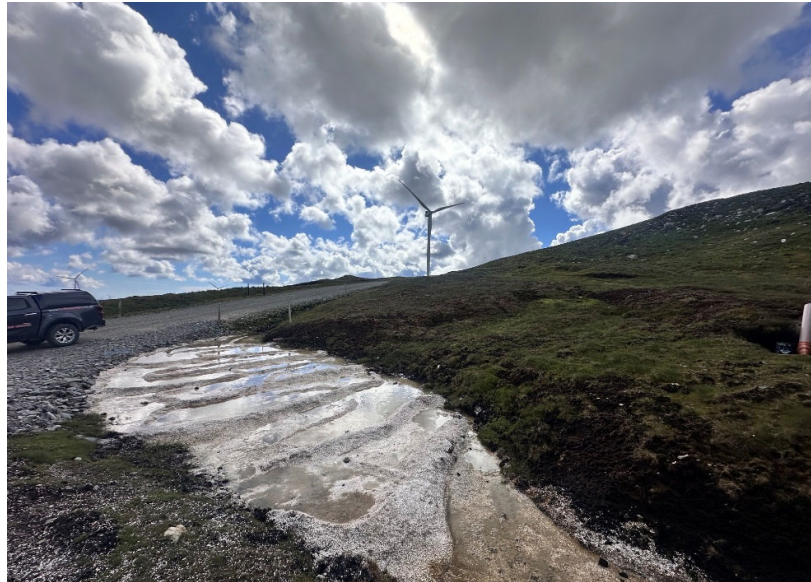
Photo 3. Existing temporary drainage treatment system downstream of KBP02
