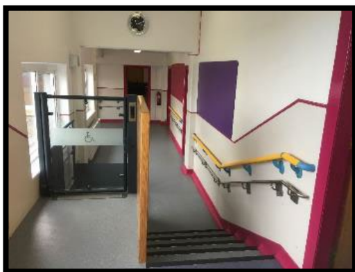
Double height handrails in contrasting colours with nosings highlighted on stairs along with an accessible lift.
