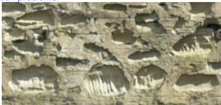
Photo of damage by incorrect cement pointing to an historic building in Lerwick (photo by A Taylor)
