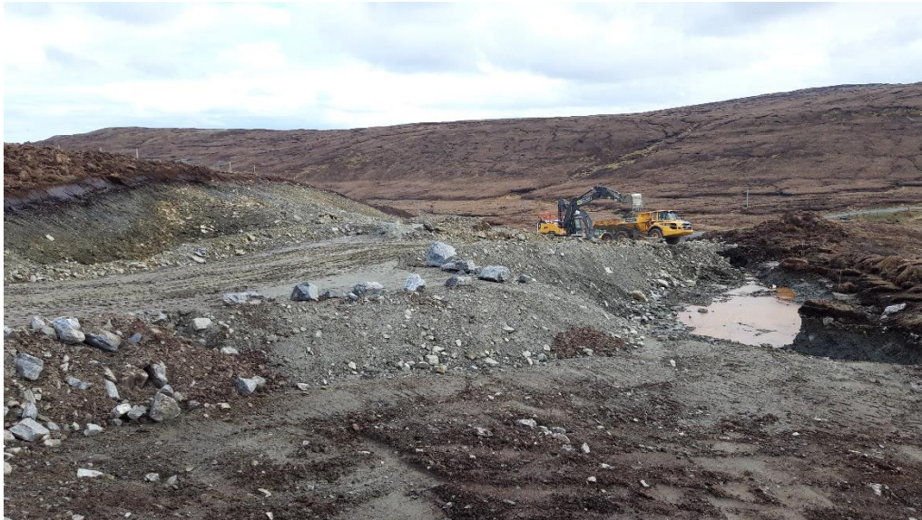
Photo 9. Excavation of rock at Hamarigrind Scord, being removed for use at the crane pad hardstanding for K78.
