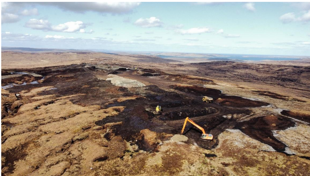
Photo 18. Aerial view of peat restoration area P27 in the foreground, and borrow pit NBP05 in the background.
