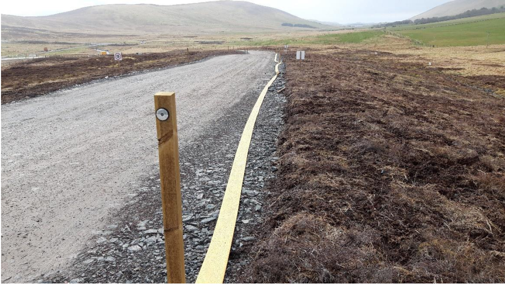
Photo 3. Perforated pipes along KAT for dust mitigation. Pump located in distance.
