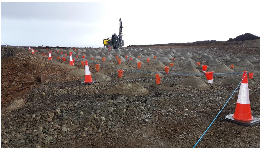
Photo 16. Drilling rig working in borrow pit NBP05, preparing for the next blast.
