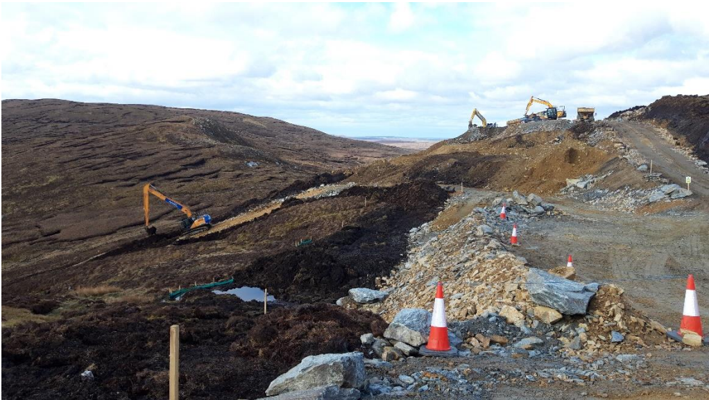
Photo 4. View of peat slip area at CH2450 of Spur 4 at Kergord. Recovery of peat and slope stabilisation in progress.
