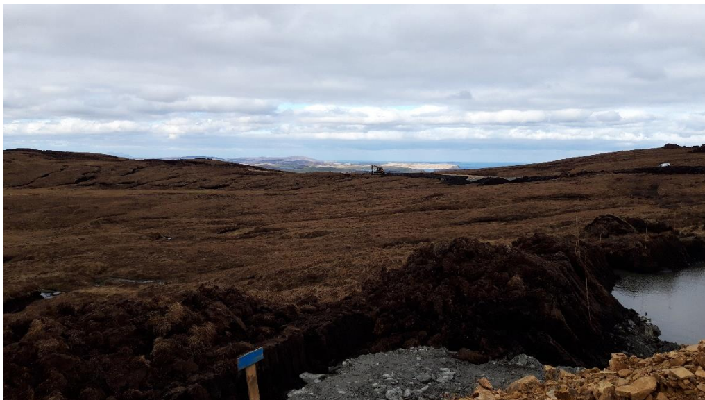
Photo 2. View of activity in peat restoration area P05 from crane pad hardstanding of K54.
