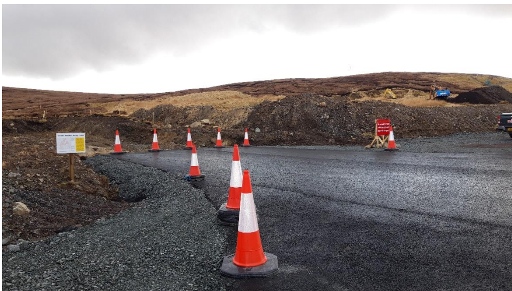
Photo 10. Access point for North Compound at the junction with the A970. Excavators in the background are progressing construction of the North Compound platform.
