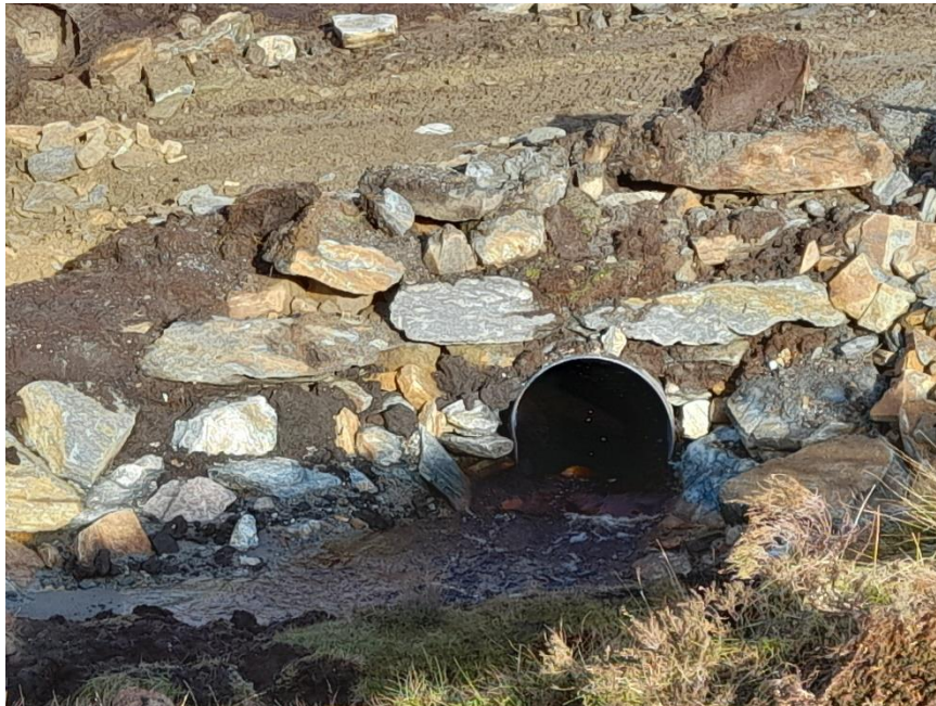
Photo 6. Stone lined gully and covered culvert in the Burn of Weisdale diversion
