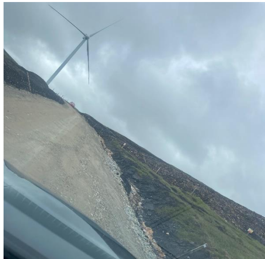
Photo 6. Drains on spur 5 between KBP02 and junction 13
