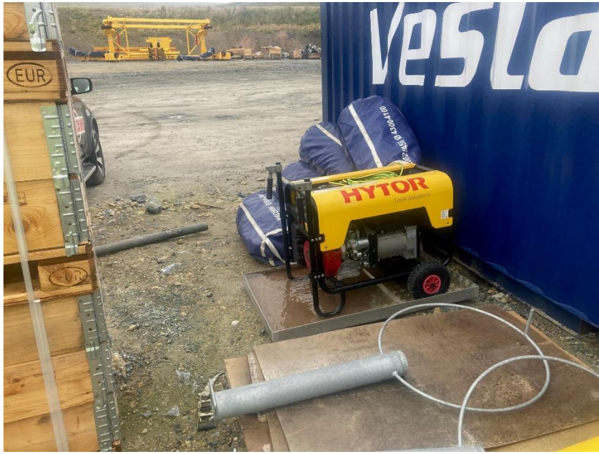
Photo 11. Open drip tray at Vestas North compound
