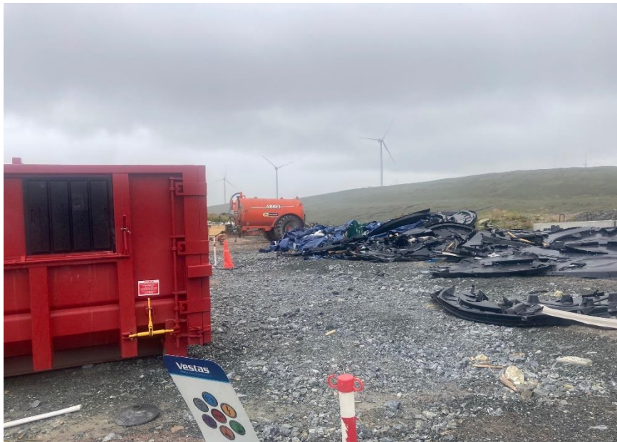
Photo 12. Loose plastic waste at Vestas North Compound
