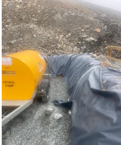
Photo 3. Damaged wall of bundled area plastic sheeting within Vestas Satellite compound at KBP05
