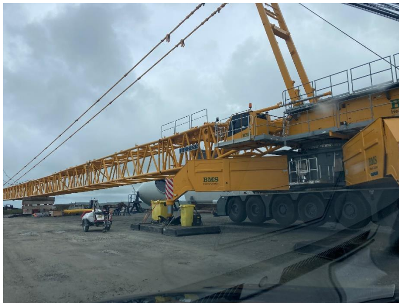
Photo 16. Crane at T075 with spill kits in place and turbine components at the base waiting to be lifted
