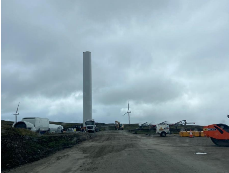
Photo 15. View of partial construction at T069, with turbine components at the base
